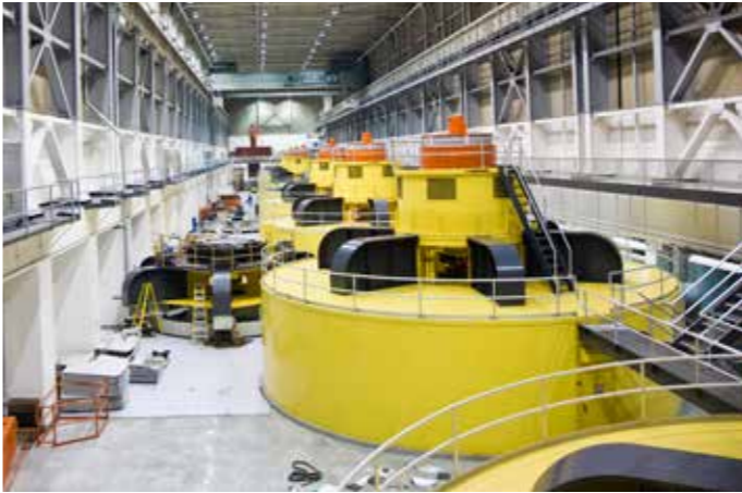
Hydroelectric power generators
